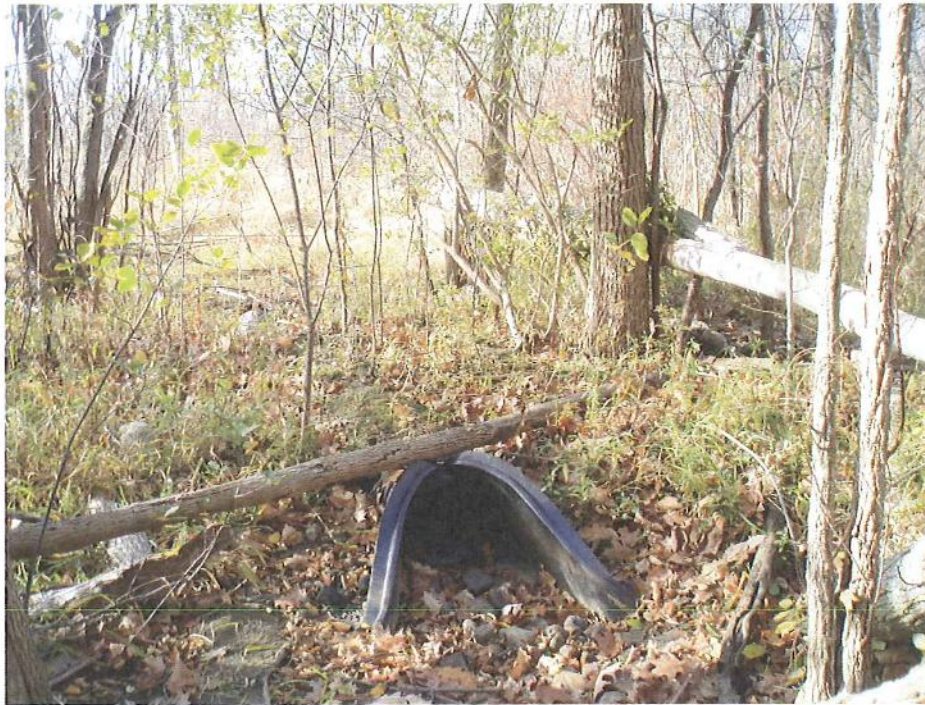
8) Drain pipe connecting to Wetland E.
